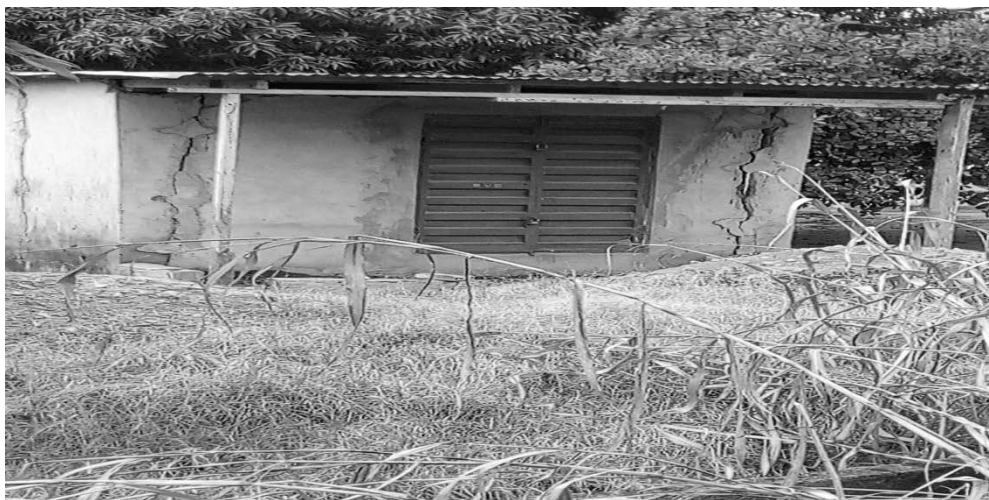
Fig. 1: Showing a Shop Affected by Industrial Blasting at Ewekoro, Nigeria.
